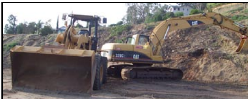
Construction on the new Lakeside Fire Protection District site at 12216 Lakeside Avenue in Lakeside. Photo credit: Patt Bixby
