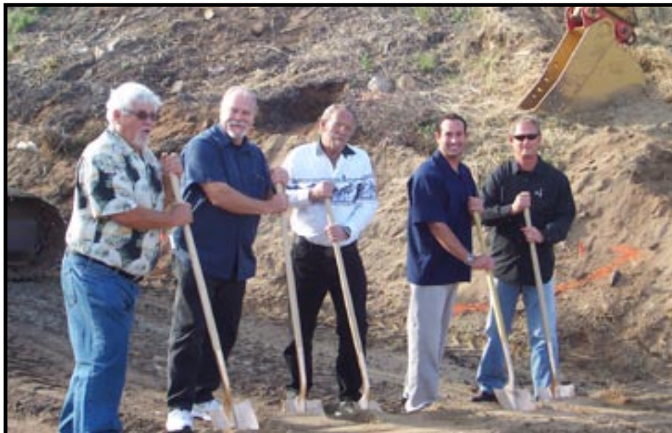
(L-R) P. Liebig, K. Coyle, Chair R. Smith, N. Johnson and J. Bingham break ground on the new Lakeside Fire Protection District. Photo credit: Patt Bixby
